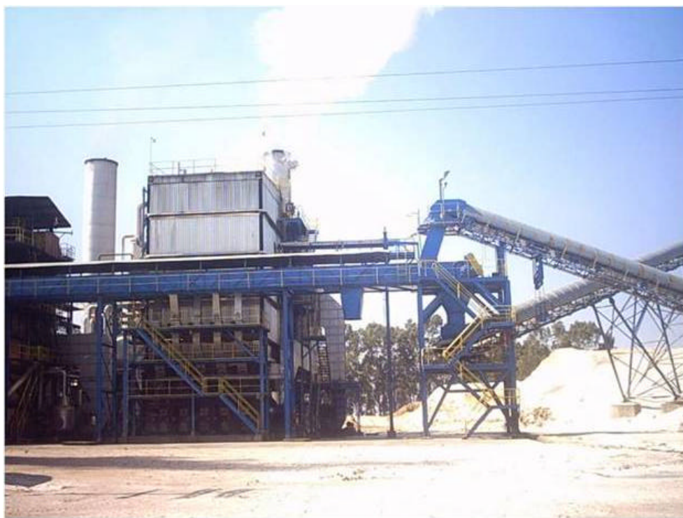
View of the current boiler / generation facilities
