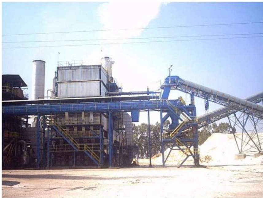
View of the current boiler / generation facilities (source: Unialco S.A.)
