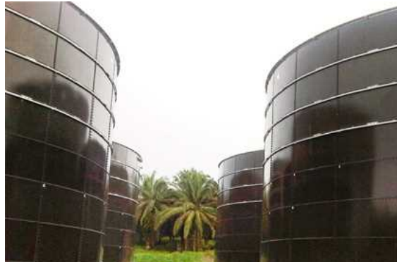
Sandakan, Sabah, Malaysia FFB 90Mt/hr > 3MW
