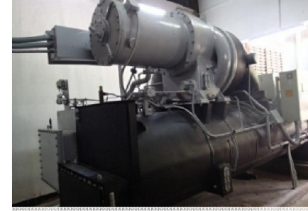
High efficiency air-conditioning and process cooling, Ebara refrigeration equipment & systems, Indonesia
