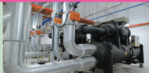
Chiller & LED Lighting (Vietnam) Tokyu Corporation
