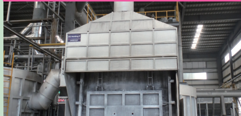
High Efficiency Furnace System (Thailand) Daiki Aluminium Industry Co., Ltd.
