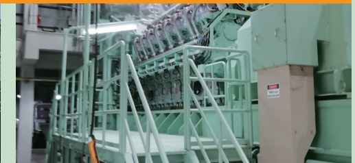
Gas Co-generation System & Chiller (Thailand) The Kansai Electric Power Co., Inc.
