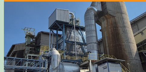
ORC Waste Heat Recovery Power Generation (Thailand) AGC Inc.
