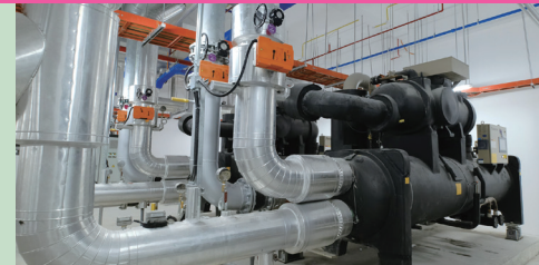
Chiller & LED Lighting (Vietnam) Tokyu Corporation
