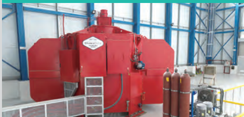
Mini Hydro Power Plant (Philippines) Toyota Tsusho Corporation
