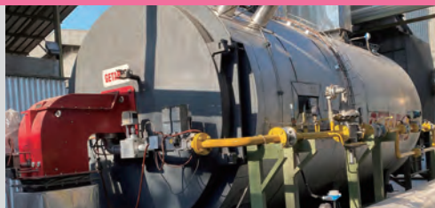
Thermal Oil Heater System (Indonesia) Fumakilla Limited
