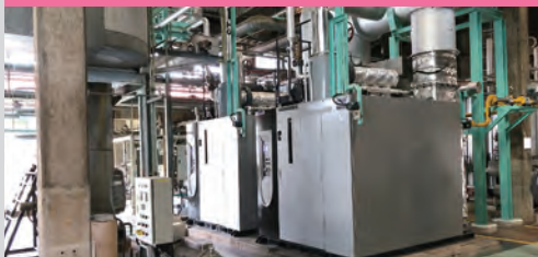
Boiler & Chiller & Solar Power (Thailand) The Kansai Electric Power Co., Inc.
