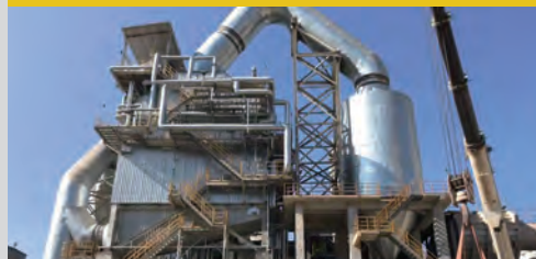
Waste Heat Recovery (Myanmar) Global Engineering Co., Ltd.
