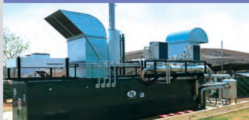
Power Generation with Methane Gas Recovery System (Mexico) NTT Data Institute of Management Consulting, Inc.
