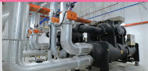
Chiller & LED Lighting (Vietnam) Tokyu Corporation
