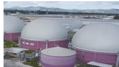
Biogas Power Generation, ITOCHU Corporation, Philippines
