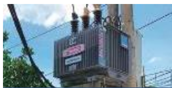
Amorphous transformers in power distribution, Yuko-Keiso, Vietnam
