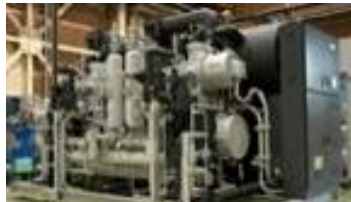
High-efficiency refrigerator, Mayekawa MFG, Indonesia
