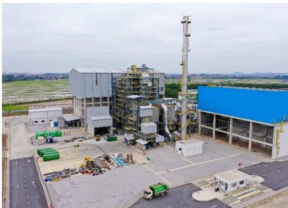
Waste to Energy Plant, JFE engineering, Viet Nam
