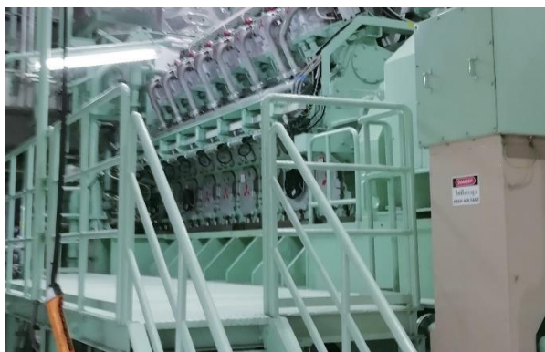
Gas Co-generation System and Absorption Chiller, Kansai Electric Power, Thailand
