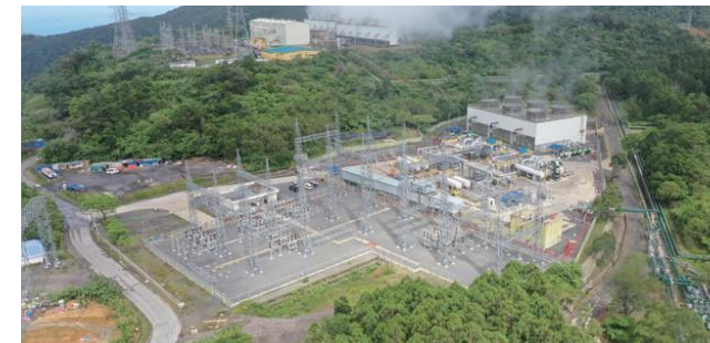
Binary Geothermal Power Generation (Philippines) Mitsubishi Heavy Industries, Ltd.
