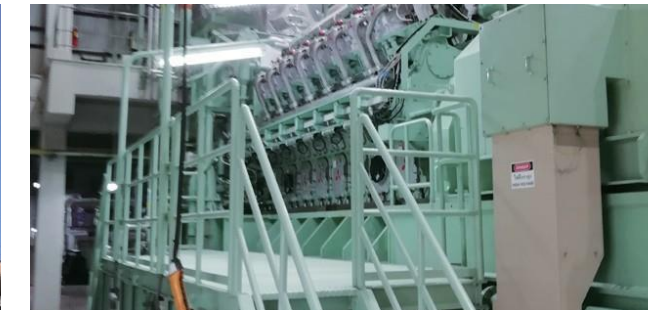
Gas Co-generation System & Chiller (Thailand) The Kansai Electric Power Co., Inc.
