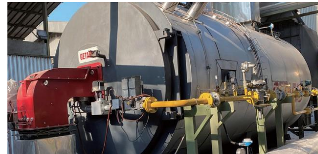
Thermal Oil Heater System (Indonesia) Fumakilla Limited
