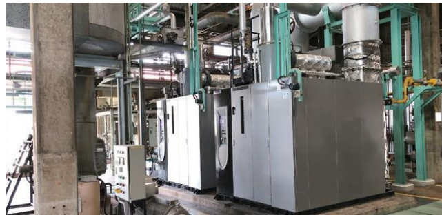
Boiler & Chiller & Solar Power (Thailand) The Kansai Electric Power Co., Inc.
