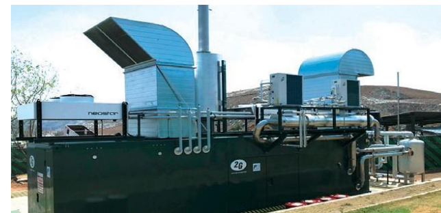
Power Generation with Methane Gas Recovery System (Mexico) NTT Data Institute of Management Consulting, Inc.
