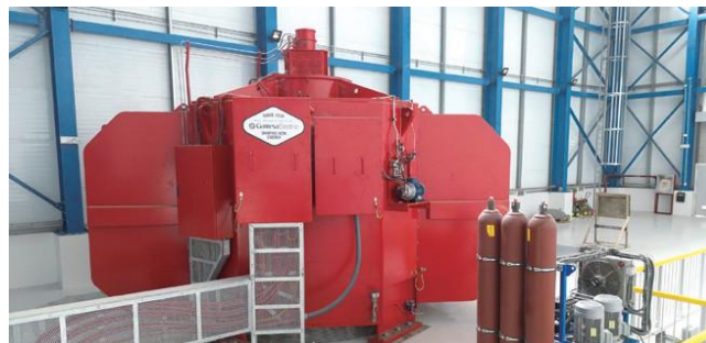
Mini Hydro Power Plant (Philippines) Toyota Tsusho Corporation
