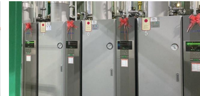
Once-through Boiler (Indonesia) DIC Corporation
