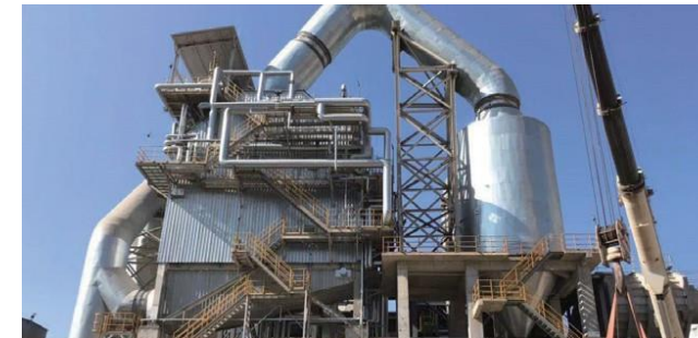
Waste Heat Recovery (Myanmar) Global Engineering Co., Ltd.
