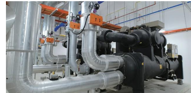
Chiller & LED Lighting (Vietnam) Tokyu Corporation
