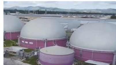
Biogas Power Generation, ITOCHU Corporation, Philippines
