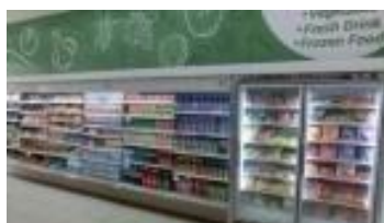
Energy saving at convenience stores, Panasonic, Indonesia
