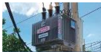
Amorphous transformers in power distribution, Yuko-Keiso, Vietnam
