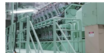
Gas Co-generation System and Absorption Chiller, Kansai Electric Power, Thailand
