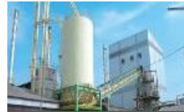
Biomass Co-Generation System, Fuji-Foods Corporation, Thailand
