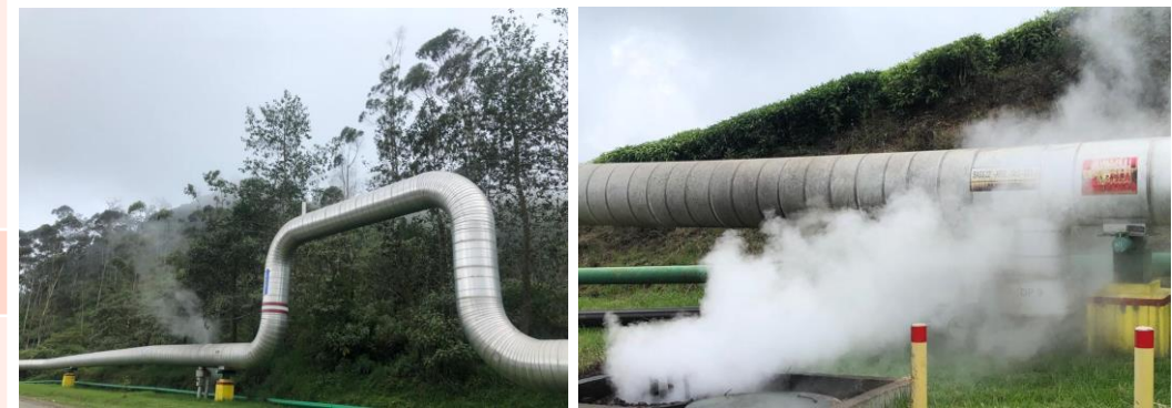
Geothermal steam pipes
