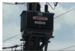
Amorphous transformers in power distribution, Hitachi Materials, Vietnam
