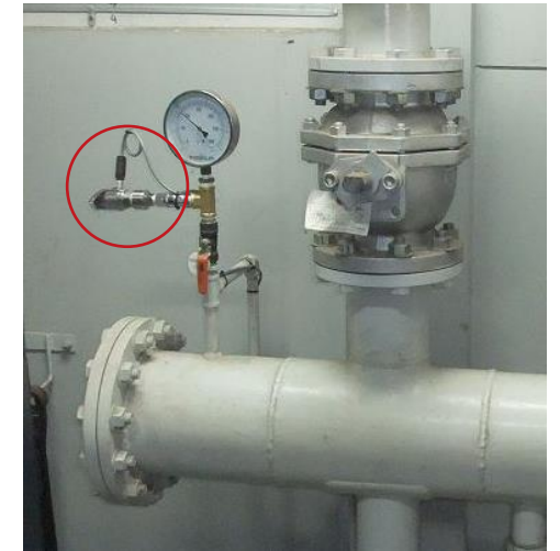
Pressure sensor installation
