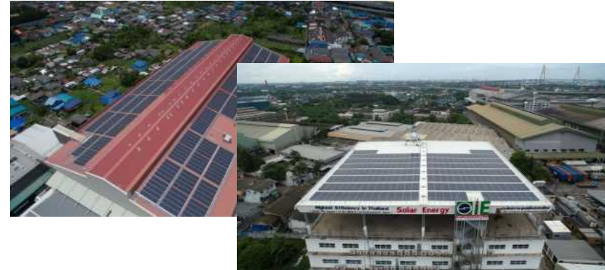
Introduction of Solar PV System on Factory Rooftop (Thailand)
