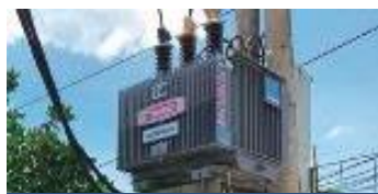
Amorphous transformers in power distribution, Yuko-Keiso, Vietnam
