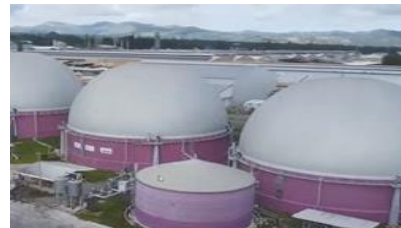
Biogas Power Generation, ITOCHU Corporation, Philippines
