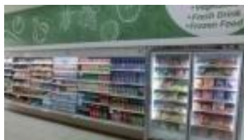
Energy saving at convenience stores, Panasonic, Indonesia
