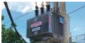
Amorphous transformers in power distribution, Yuko-Keiso, Vietnam
