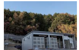
No.19-5 Hybrid Autonomous Power Control System with Renewal Energy
