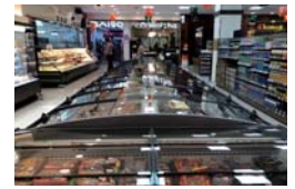
No.20-2 High-performance ventilation, air conditioning, and showcase combined control to Food Supermarket
