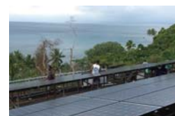
Small Scale Solar Power Generation (Palau)
