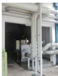
A chiller for plant air conditioning and process cooling systems (Indonesia)
