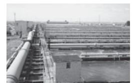
Waste Water Treatment Plant (Shimizu Corp.)
