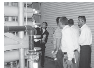
Field trip to small waterworks facility using the reverse osmosis process in Maibara City
