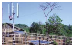
Photovoltaic and wind power generation apparatus (Marubeni Corp.)
