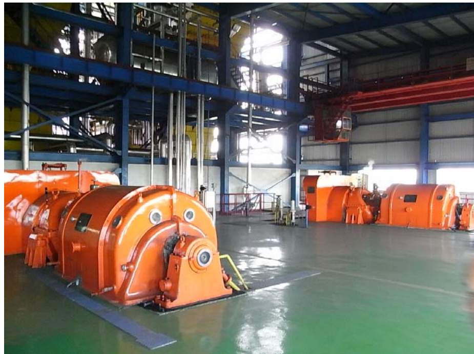
Figure 3: Steam Turbine Generator
