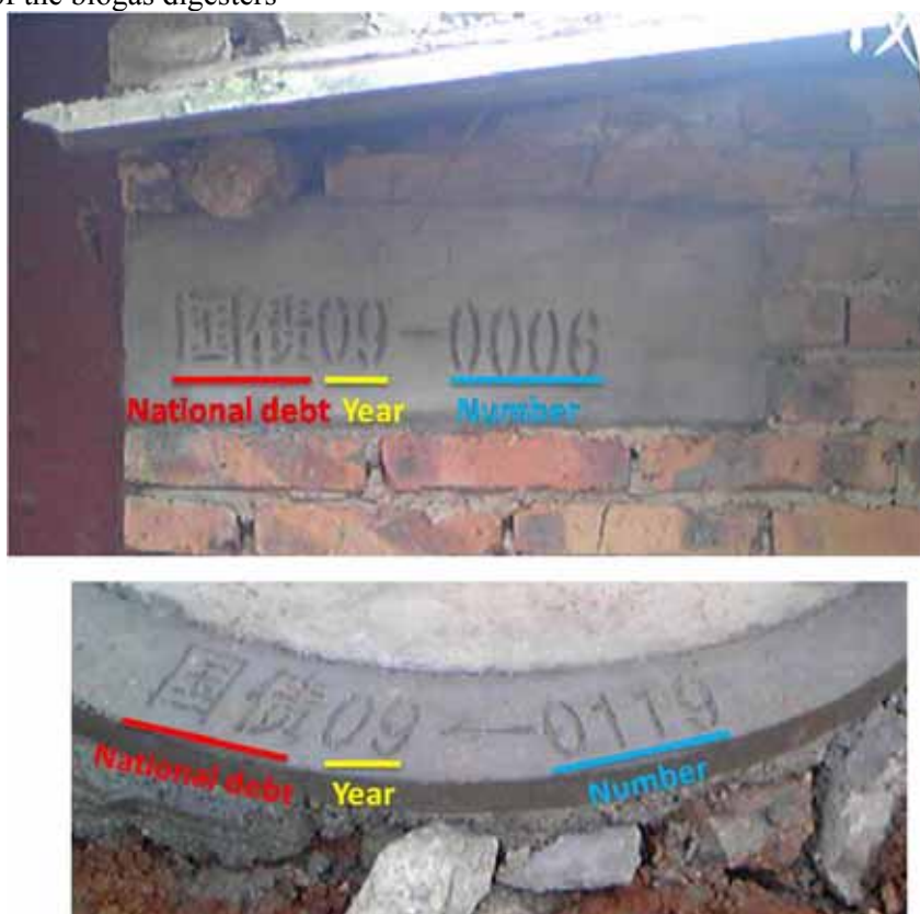
Figure 3 Mark of biogas digesters
