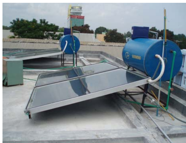
Figure 2. SWH system with flat plate solar collectors
