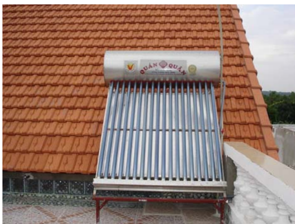
Figure 1. SWH system with evacuated tube solar collectors
