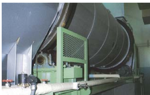
Photo-1 Sludge dryer
