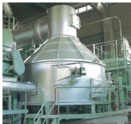
Photo-2 Vortex Incinerator
