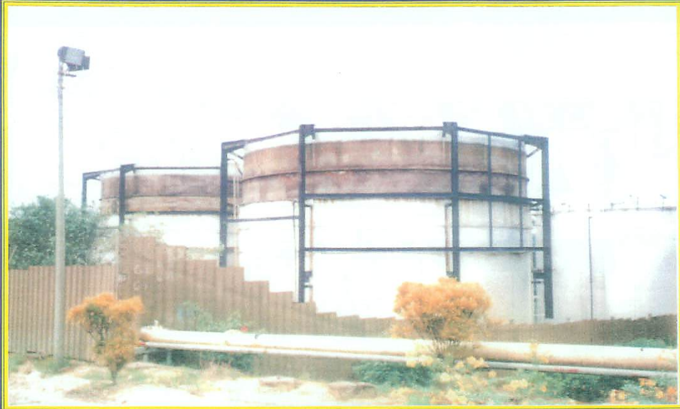
A View of the Floating Top Closed-Tank Anaerobic Digester
