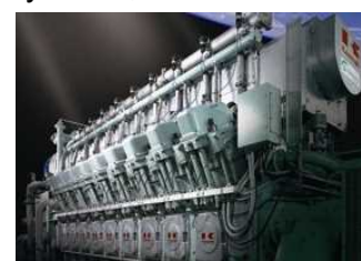
Co-generation system at factory, Toyota, Nippon Steel & Sumikin Engineering, Indonesia, Thai
