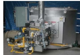
Regenerative Burners in industries, Toyotsu Machinery, Indonesia
