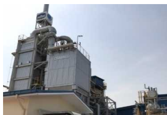
Waste to Energy Plant, JFE engineering, Myanmar
