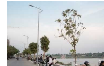
LED street lighting system with wireless network control, MinebeaMitsumi, Cambodia
