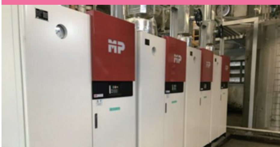
Once Through Boiler (Thailand)
