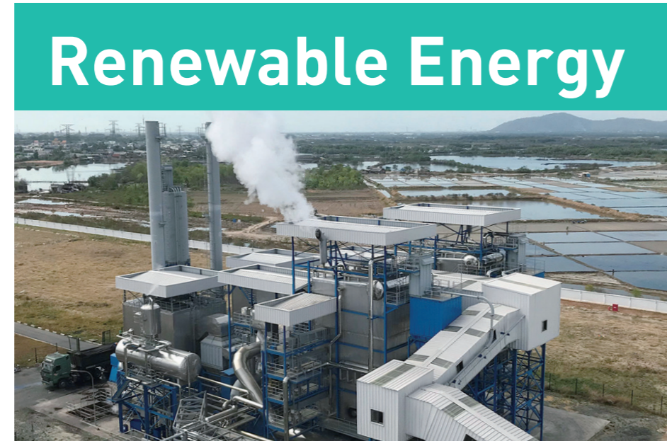
Biomass Boiler (Vietnam)
