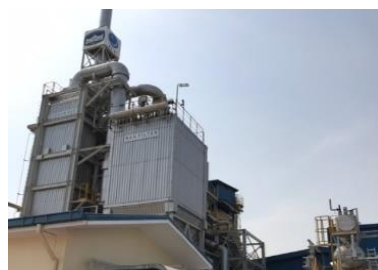
Waste to Energy Plant, JFE engineering, Myanmar
