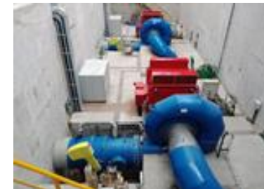
Hydro Power Plant, Chodai Co., Ltd., Philippines
