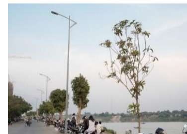
LED street lighting system with wireless network control, MinebeaMitsumi, Cambodia
