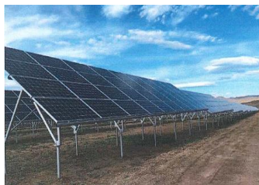
Solar power, Farmdo Co., Ltd., Mongolia
