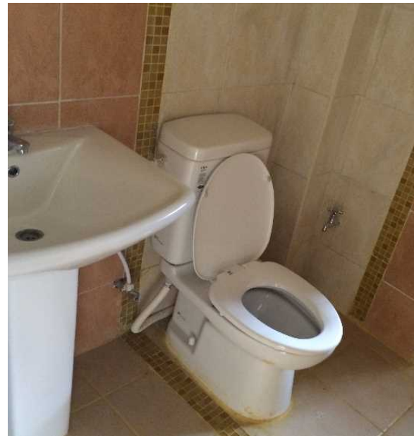
Figure 2 : Installed Micro Flush Toilet
