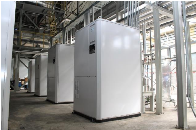
Heat recovery heat pumps
