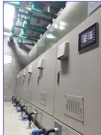
Picture of the Heatpump in the AXIA
