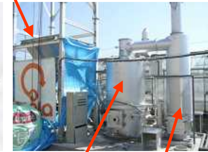
Furnace & heat exchanger
