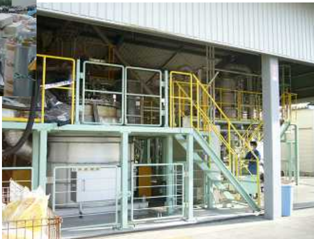
Liquid fuel production plant in a waste generation site
