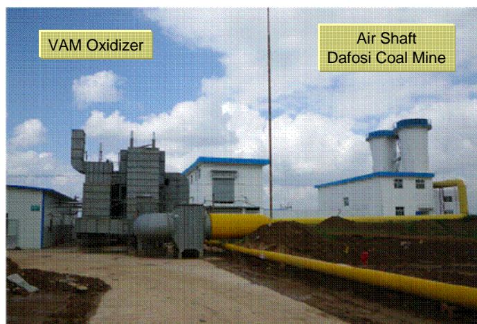
Figure 3-3 VAM Oxidizing System at Dafosi Coal Mine for full scale field trial.
