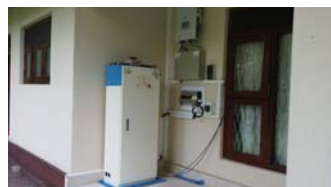
No.17-7 Energy Storage System_5kWh
