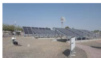
No.17-11 High performance solar power generation system adopted to desert conditions.
