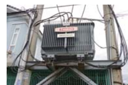
No.15: Introduction of Amorphous high efficiency transformers in power distribution systems (Vietnam)
