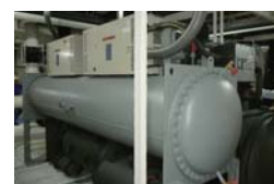
No.15: Energy Saving for Semiconductor Factory with High Efficiency Centrifugal Chiller and Compressor (Chiller)
