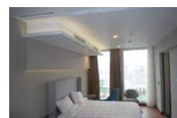
No.17: Introduction of High Efficiency Air-Conditioning in a Hotel (units installed in the guest rooms).
