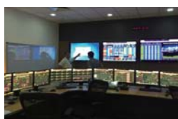
No. 14-4: Central monitor room for a district cooling plant (an optimum control system is planned to be installed)
