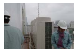
No.17: Introduction of High Efficiency Air-Conditioning in a Hotel (outdoor air-processing units installed in the terraces).
