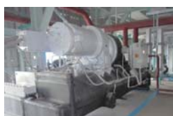
No.1: Energy saving for air conditioning & facility cooling by high-efficiency centrifugal chiller (Bangladesh)
