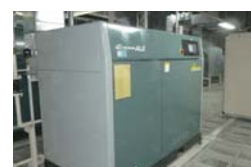
No.15: Energy Saving for Semiconductor Factory with High Efficiency Centrifugal Chiller and Compressor (Compressor)
