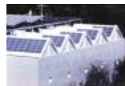
Solar power generation panels installed on the roof of the UNEP-IETC Osaka Centre
