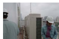
No.17: Introduction of High Efficiency Air-Conditioning in a Hotel (outdoor air-processing units installed in the terraces).
