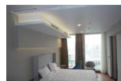
No.17: Introduction of High Efficiency Air-Conditioning in a Hotel (units installed in the guest rooms).
