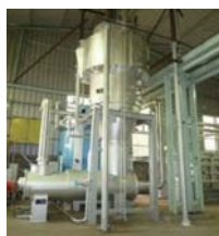
No. 15-5: Superheated steam generator and Dry distillation gas combustion equipment
