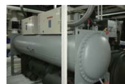
No.15: Energy Saving for Semiconductor Factory with High Efficiency Centrifugal Chiller and Compressor (Chiller)
