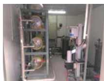
No. 15-2: Seawater desalination system (Reverse Osmosis (RO) module with hollow fibre Reverse Osmosis membrane)
