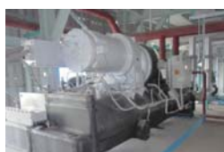
No.1: Energy saving for air conditioning & facility cooling by high-efficiency centrifugal chiller (Bangladesh)
