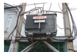
No.15: Introduction of Amorphous high efficiency transformers in power distribution systems (Vietnam)
